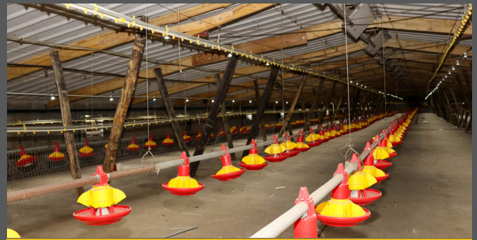
Renovations are in full swing at the Cato Ridge Poultry Farm, which began operations in 2020. The upgrades are designed to enhance the farm's operations, expand its capacity, and accommodate more poultry farmers.
